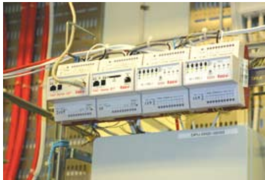
Access control and intrusion alarm is an integral part of TAC's delivery Integration and communication between climate and security systems is made possible through the Xenta 527
